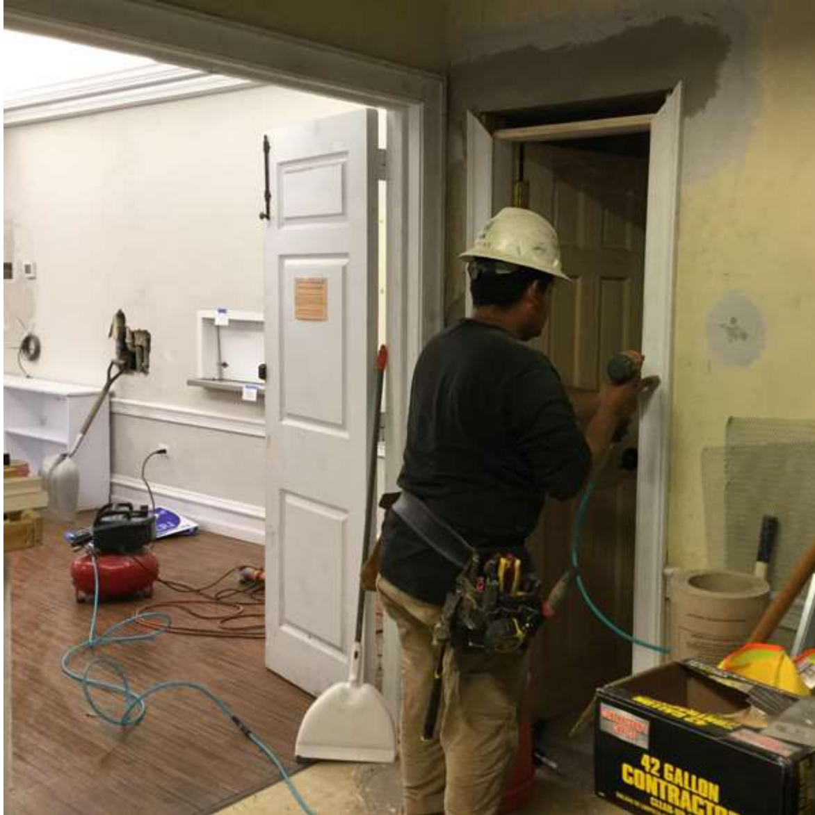
Four carpenters install a new door from the North Room to the small bathroom.
