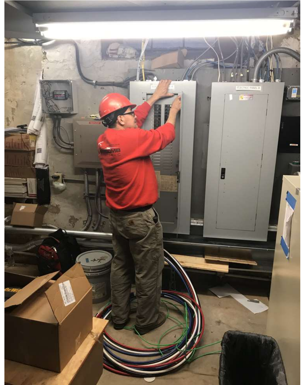
The chief electrician prepares to connect the Quaker House feeder cables to the Meeting House panel.
