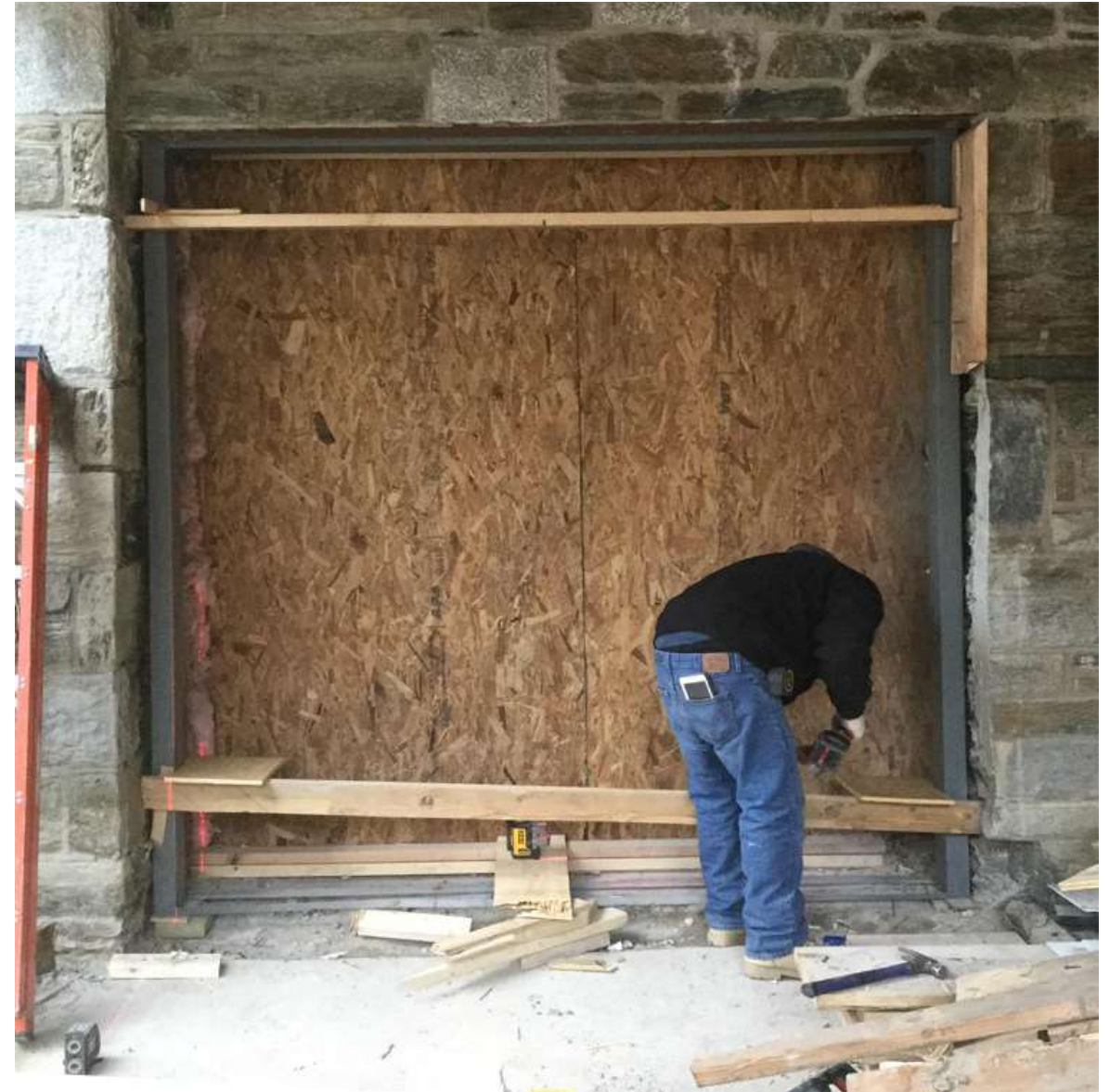
The carpenters also install a frame for the double doors that will take you from the Lobby to the Assembly Room.
